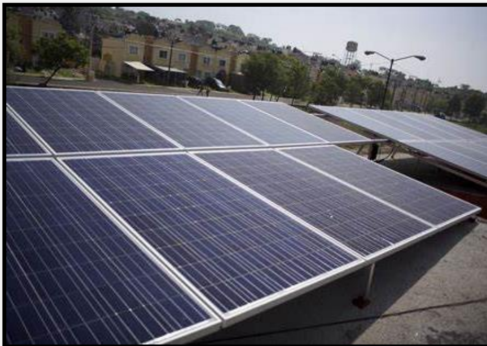
Cod 03: Panel solar
